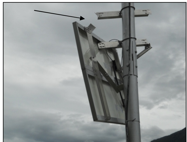
Damage to siren tower reported to the Department of Energy for reparation by contractor
